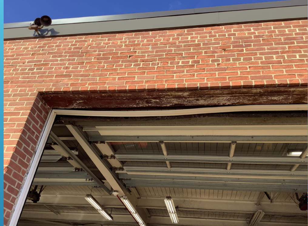
Frames are bent
