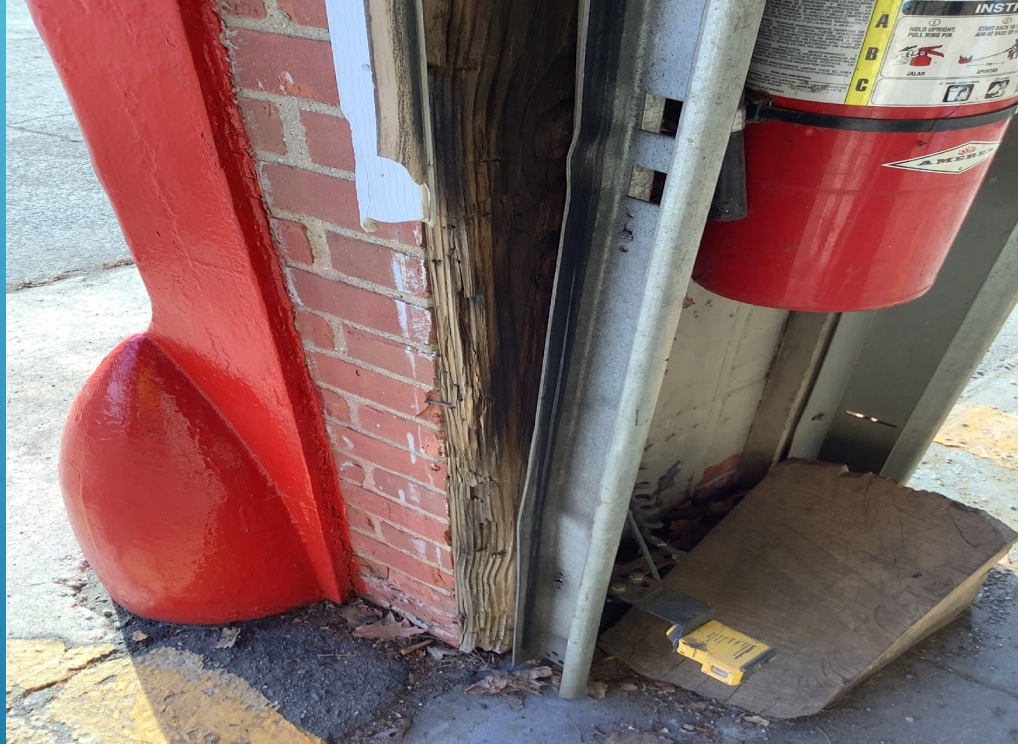
Rotted wood on doors
